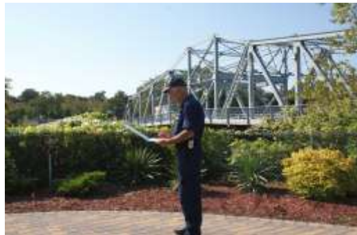
Author inspecting Gregory Ave Bridge over the Passaic River Photo: Kevin Redden
